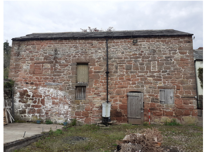
Newbiggin bank barn, a former bastle at Townhead Farm seen from the 'low' side in the farmyard. Note the small blocked windows at first floor level, and the signs of two roof raisings. (with thanks to Lee Paton and Mathias Motz).
